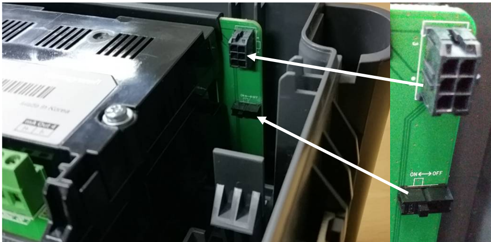
Figure 18. Battery On/Off Switch and Battery Connector
